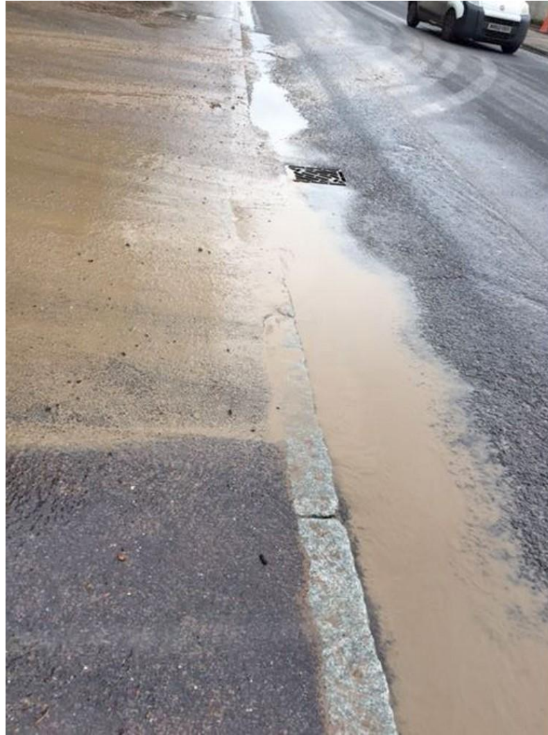
Figure 6 : Surface water runoff into Godstone Road from the Gas Holding Station
